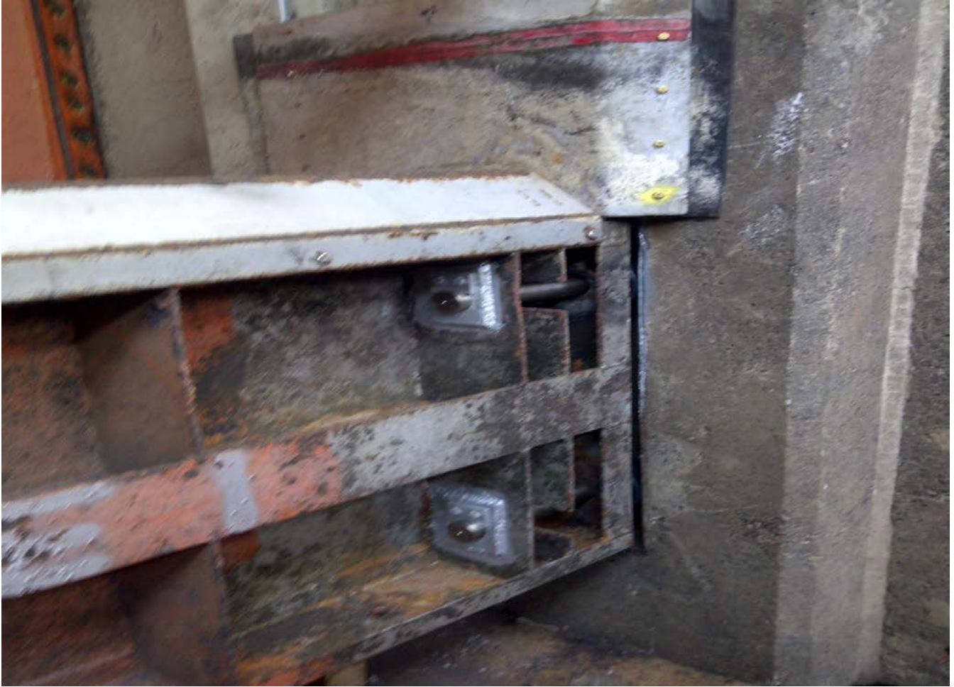
Rehabbed 159 weir with new wheels. Seals also replaced, but not visible in this pic.
